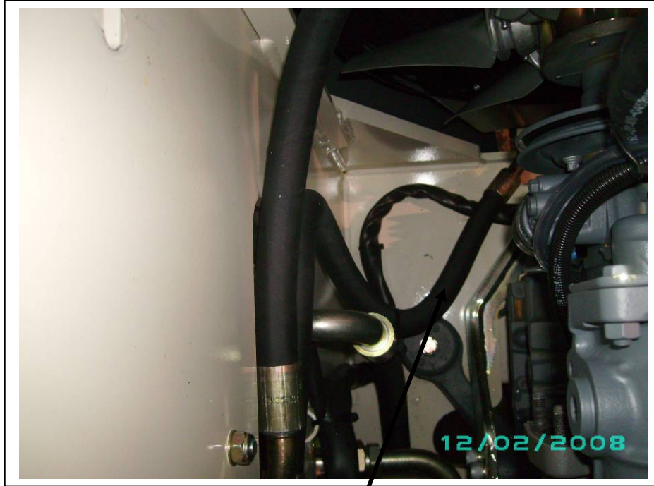
This hydraulic line must be rerouted
